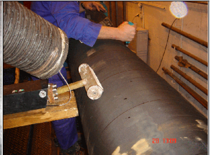
RPR Inductor mounted on platform
